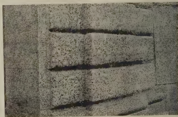
DETAIL VIEW OF ENTRANCE TO MERIDIAN HILL PARK, WASHINGTON, D. C., SHOWING EXPOSED AGGREGATE SURFACES
